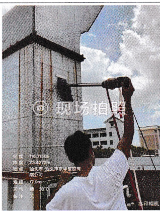
FQ-31252排气筒后
